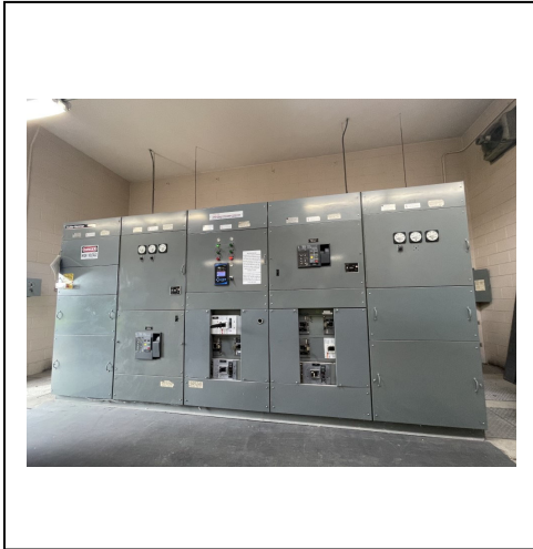
Figure 2: SWBD-1, West Generator Building
