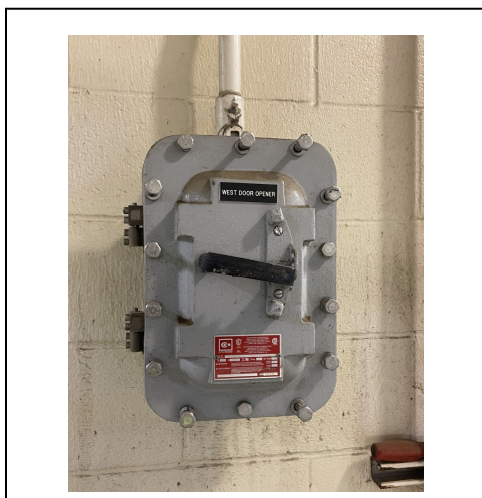
Figure 4: Explosion proof disconnect not bolted down
