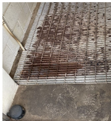
Figure 1: Metal in Grit Building
