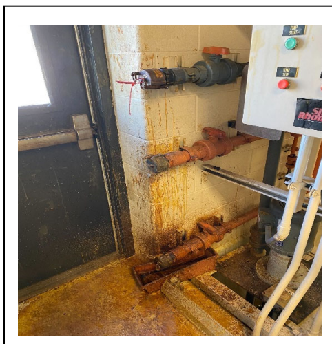
Figure 10: Ferric chloride corrosion.
