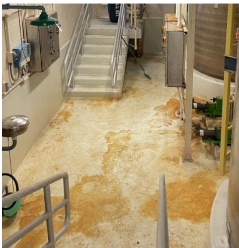
Figure 8: Ferric leaks in Filtration Building
