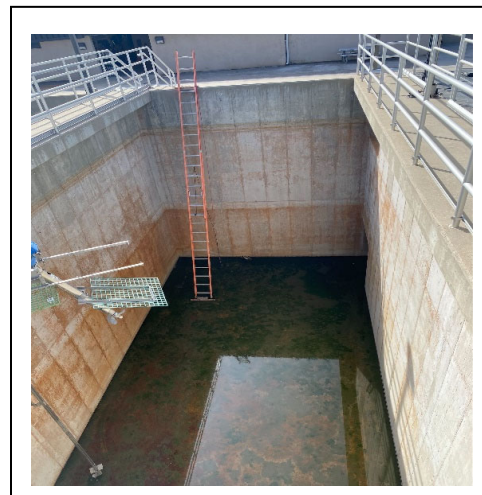
Figure 5: South Train Anoxic Basin
