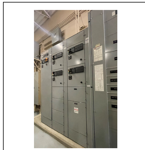
Figure 12: MCC/SWBD at reclaim pump station
