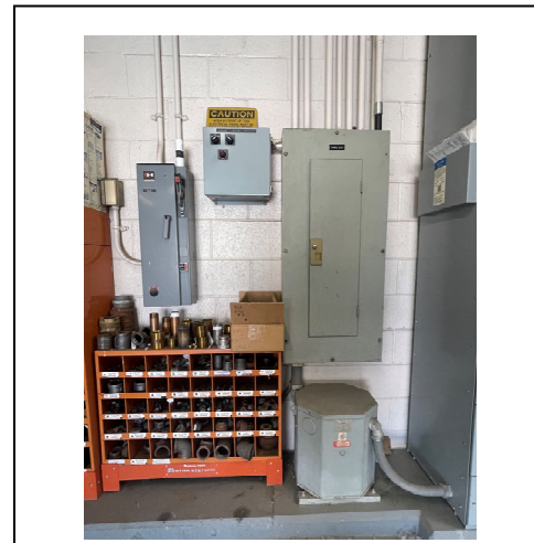
Figure 13: Panelboard EC5 and its xfmr
