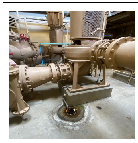
Figure 8: Seal water leaks – IR pumps
