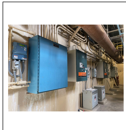
Figure 10: Five VFDs and two floor xfmr's
