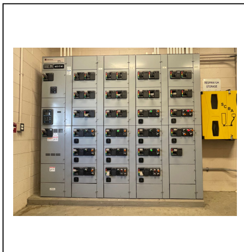
Figure 11: MCC at Reclaim Filtration Complex
