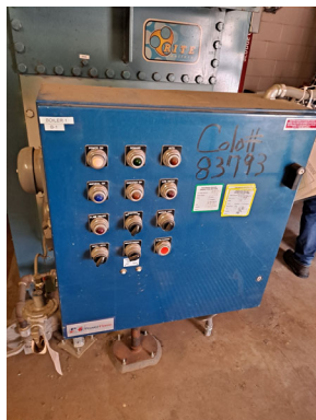
Figure 11: Boiler Control Panel
