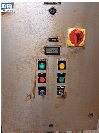
Figure 8: FCP-1 Control Panel
