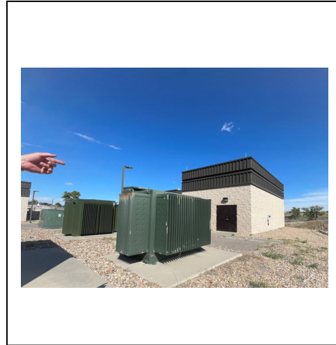
Figure 1: Two outdoor transformers
