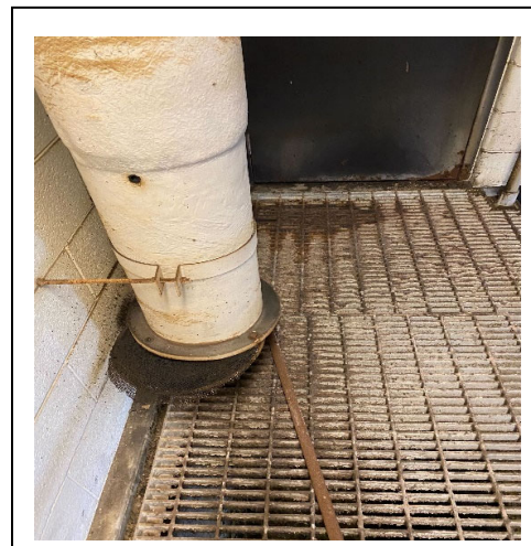
Figure 1: Clogged grit air ducts.
