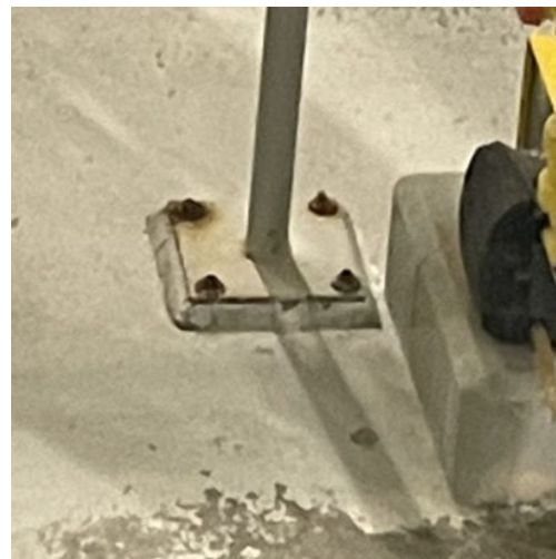
Figure 9: Corroding Anchor Rods in Hypochlorite Building
